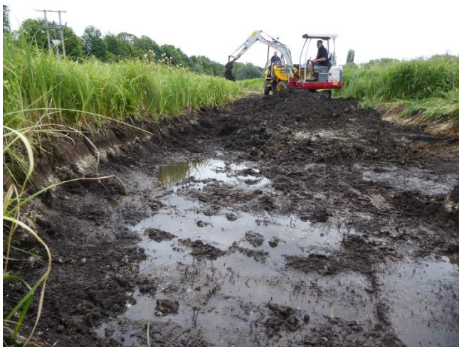
The hole started filling up with water while the digger was still working on it!
